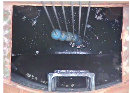
A typical float system for level control in a lift station.
